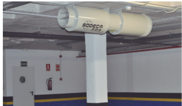
THT/IMP installed in a car park
