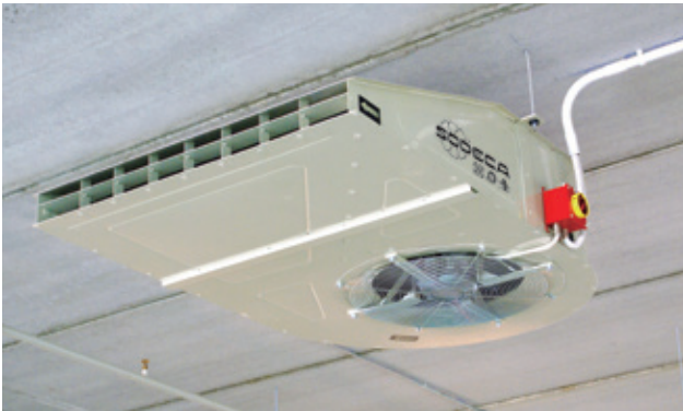
CI installed in a car park
