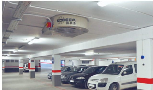
CI installed in a car park
